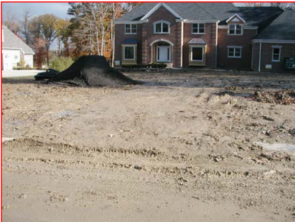
Don't. Allow sediment to discharge escape the site.
