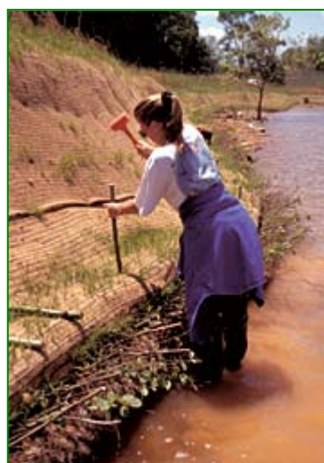
Do. Securely anchor the fiber roll to level contours with approved stakes.
