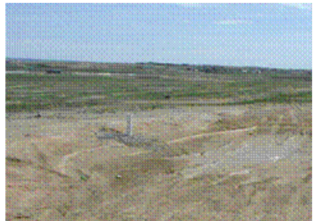
Don't. Build a sediment basin without an armored spillway.
