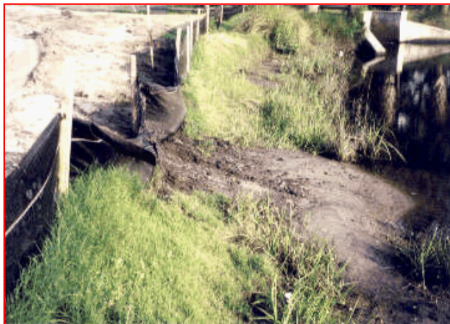
Don't. Install silt fence where flow velocity and volume will compromise structural integrity. If necessary, reinforce silt fence in sensitive areas.
