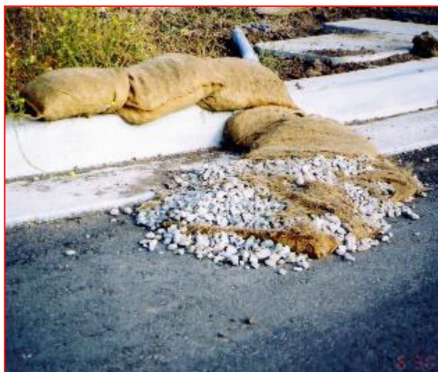
Don't. Allow bags to disintegrate and rupture spilling gravel. Gravel bag berms must be maintained to be an effective BMP.
